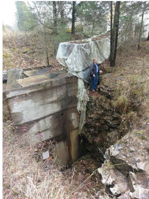
Top: Existing Greenhouse, vented with air from the cave. Bottom: Plywood façade over entrance with the wooden air duct.
