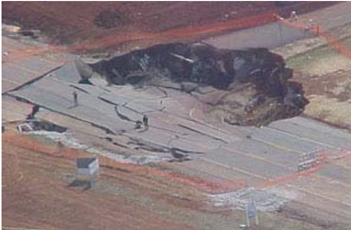
Dishman Lane Collapse into State Trooper Cave
